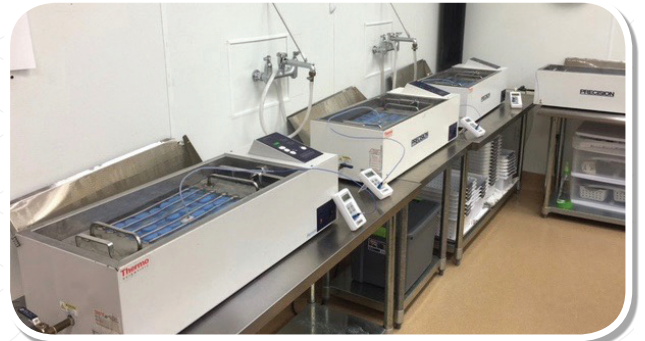
New pasteurization and sterilization room
